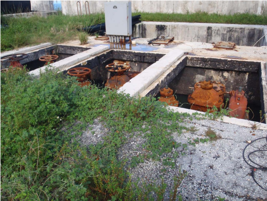
Figure 9: Malcolm Park Wastewater Treatment Plant - Pumps
