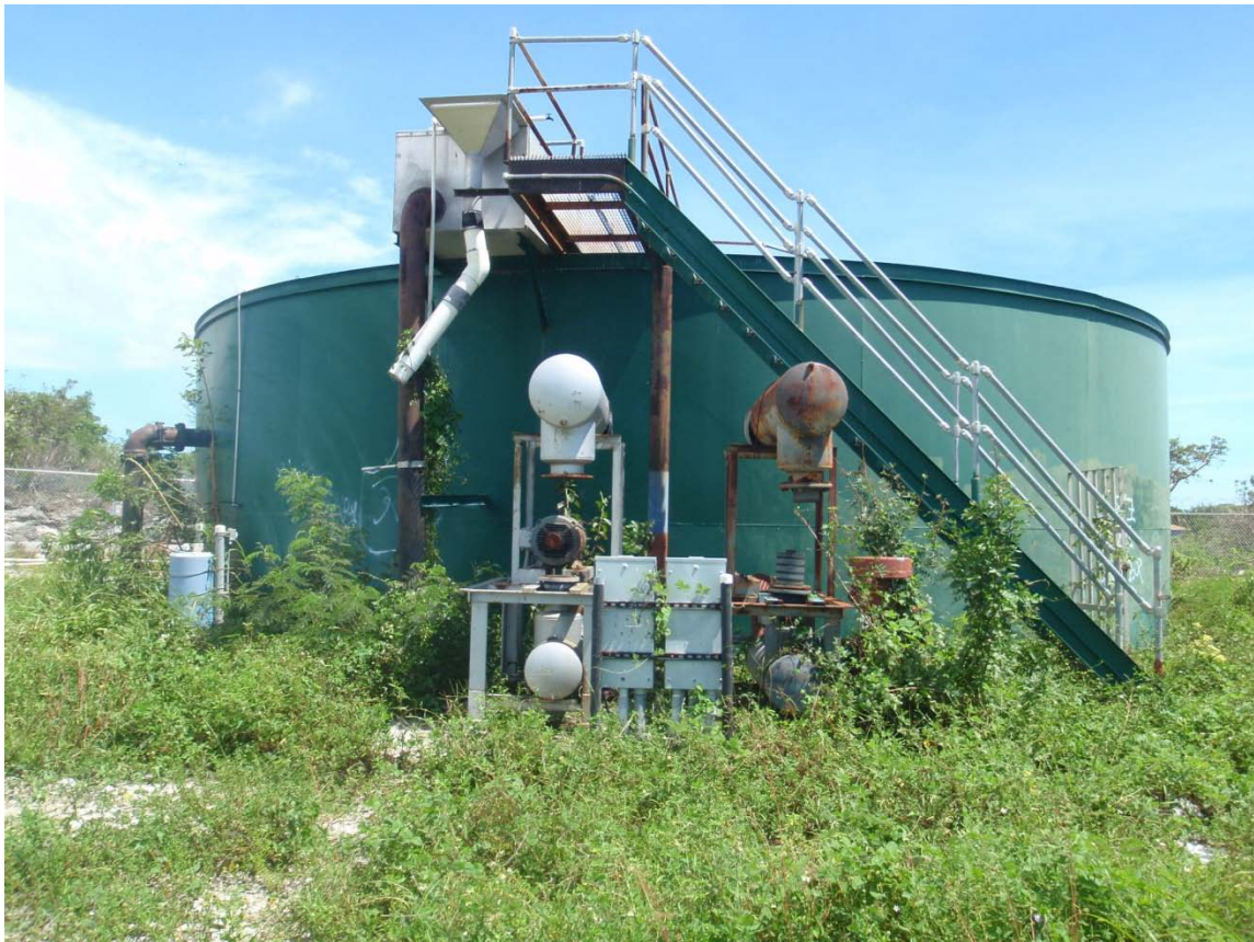
Figure 10: Flamingo Gardens Wastewater Treatment Plant
