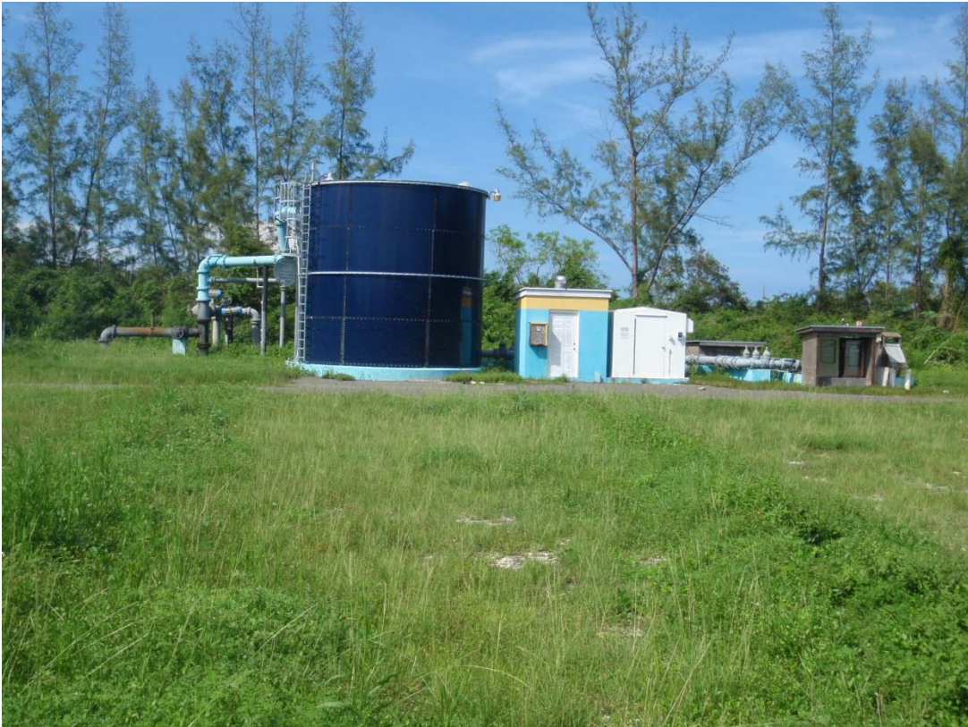
Figure 6: Fox Hill Wastewater Treatment Plant
