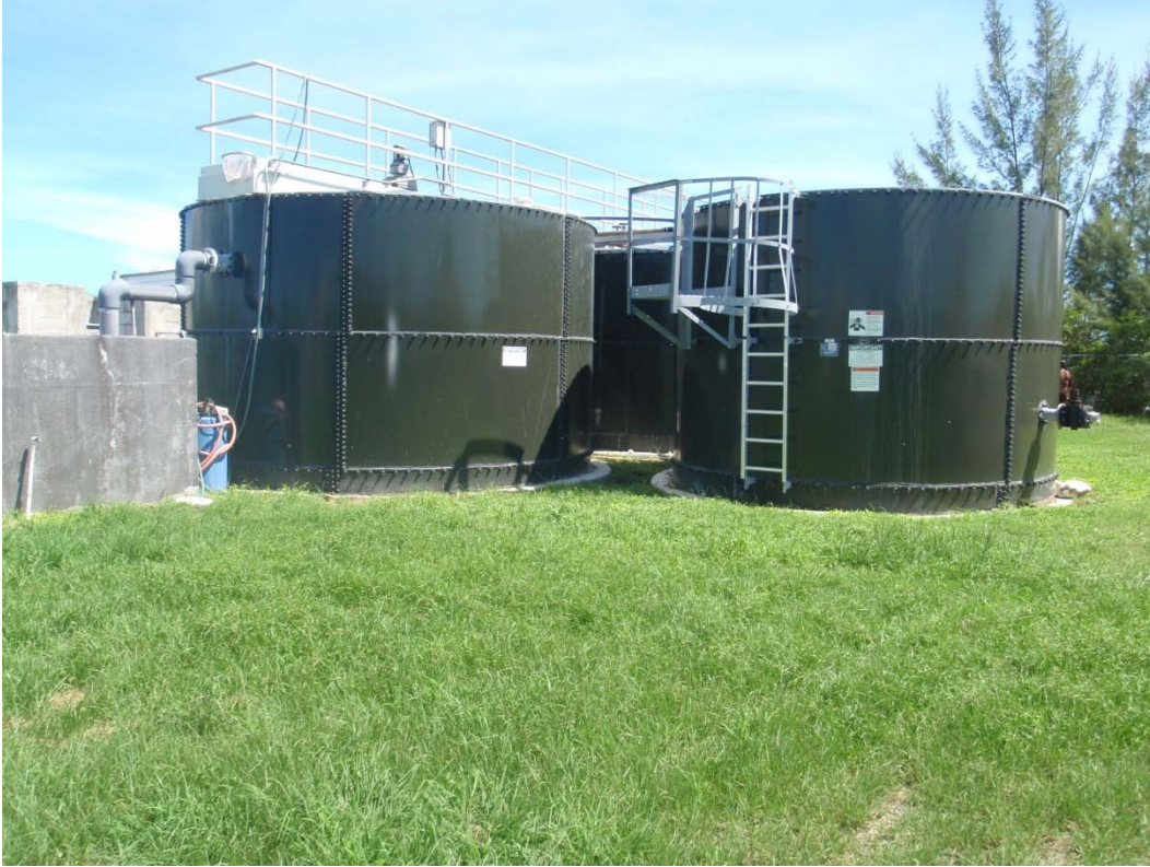
Figure 5: Coral Vista Wastewater Treatment Plant
